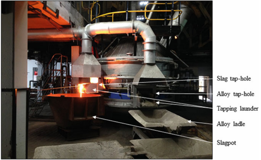
Fig. 5 Typical ladle arrangement when tapping slag from a slag tap-hole and alloy from an alloy tap-hole in bi-level arrangement
